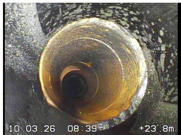
4, 00:03:15, 23.80m Rohrmaterialwechsel: Polyvinylchlorid
